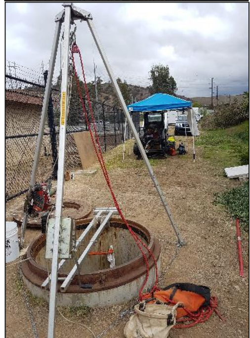
Figure 4 – PICA's skidsteer mounted winch stationed near MH #3 (top) and MH#9 (bottom). Rollers guided the winch line down into the manhole to prevent contact against abrasive surfaces and sharp edges.
