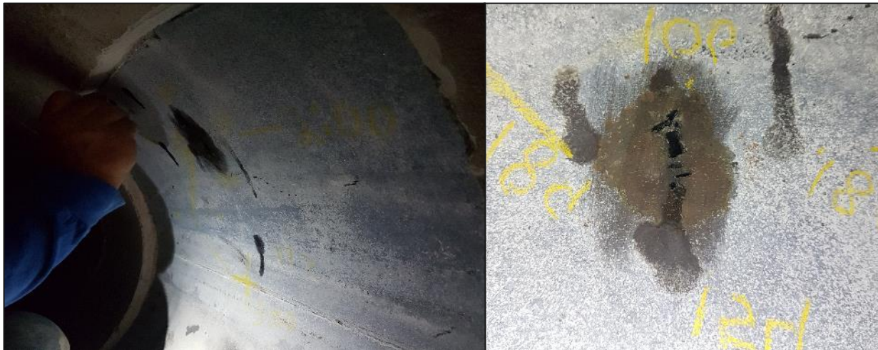
Figure A3. AWD internally exposed the reported defect location in Segment 153 (left). The reported defect location was then verified to be 100% wall loss using UT (right).
