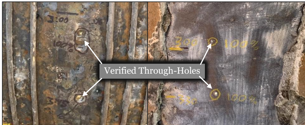
Figure A5. Segment 113 - AWD investigated the reported defect signal externally (left) and internally (right) and discovered two pinholes (100% through-holes) at this location.
