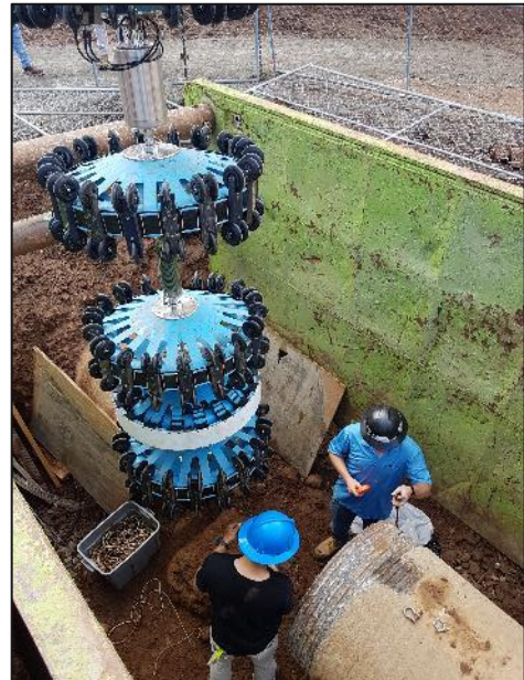
Figure 2 – The RAFT inspection tool is fully assembled above ground and lowered into the excavation where full bore pipe access is available.
