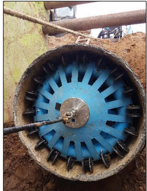
Figure 3 – The RAFT inspection tool inside the 36-inch Aqua Connector with trailing winch line attached.
