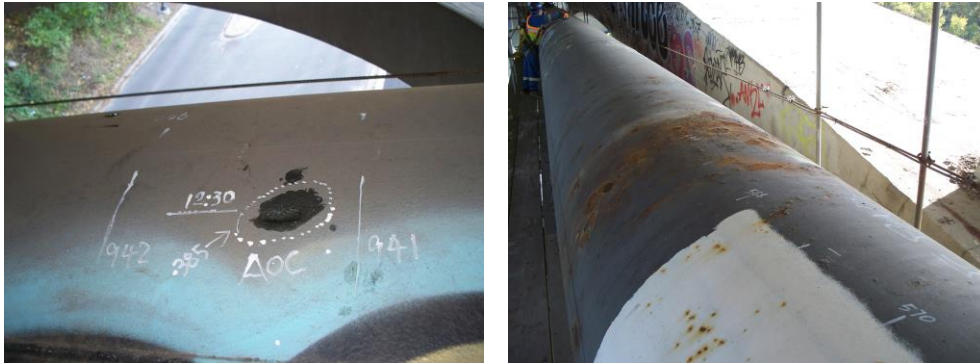
Fig 6 Local external pitting examples. The right hand photo is directly under an expansion joint of the bridge deck
