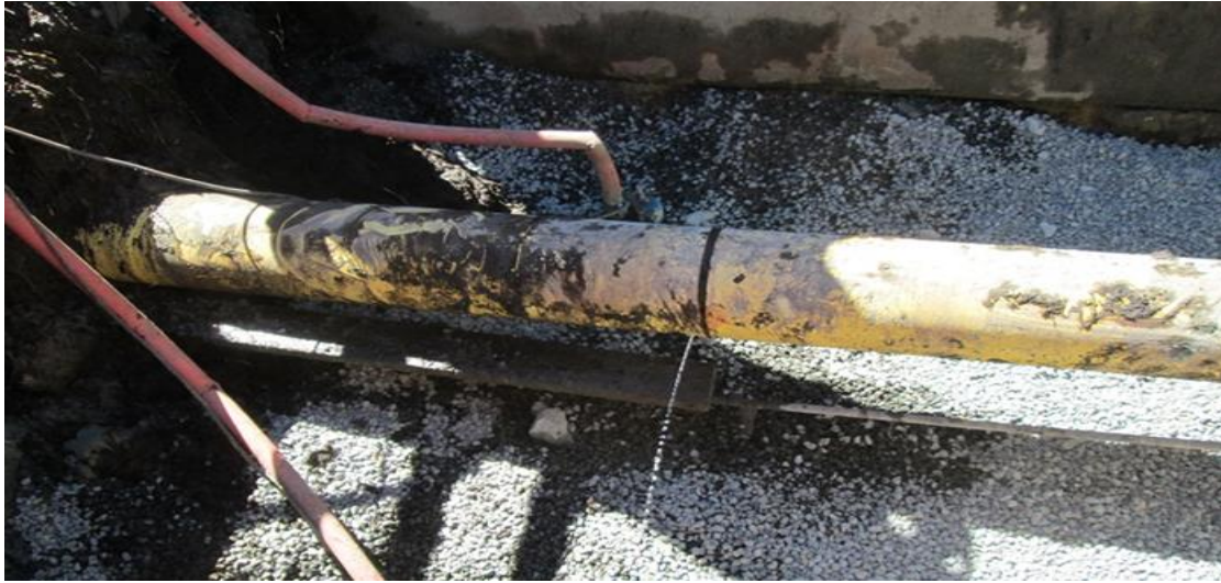
Figure 7: AOI 3a identifying a circumferential crack in pipe.
