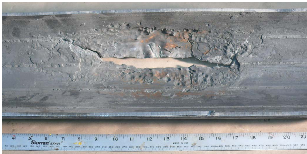
FIGURE 2 - ID of the Steel Pipe at the Failure
