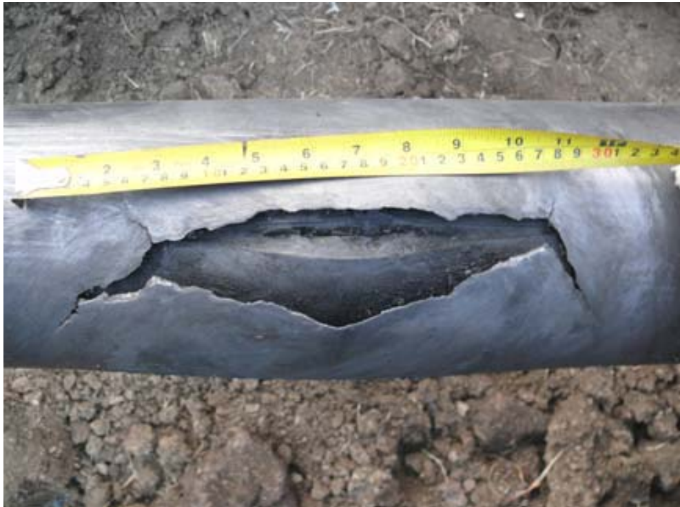
FIGURE 1 - Failure after insulation and coating removal
