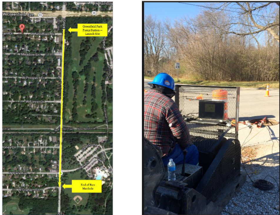
Figure 6. Aerial of Project Two (left); Receive manhole with winch and operator (right)
