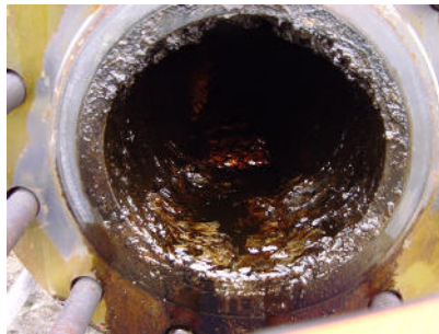
Fig-12: internal grease, sand and oil deposits
