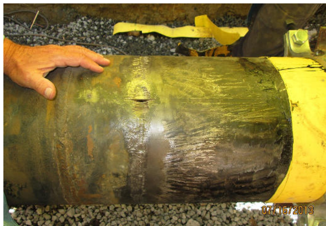
Fig-2: corrosion failure under improperly applied shrink sleeve on steel pipeline
