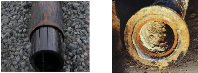
Fig-11: Showing internal liner in O&G Pipeline (left) and tubercles in cast iron water pipe (right)
