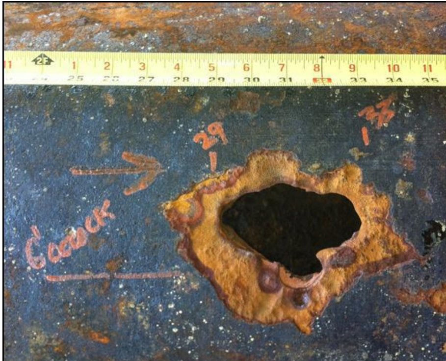
Figure 5: The through-hole located in Pipe 0030. While sludge and backfill had prevented any leaks here to date; the integrity of the pipe had been compromised due to corrosion.
