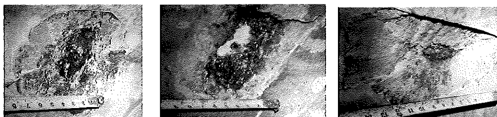
Figure 5. Areas of spalled mortar lining and exposed/corroded steel cylinders
