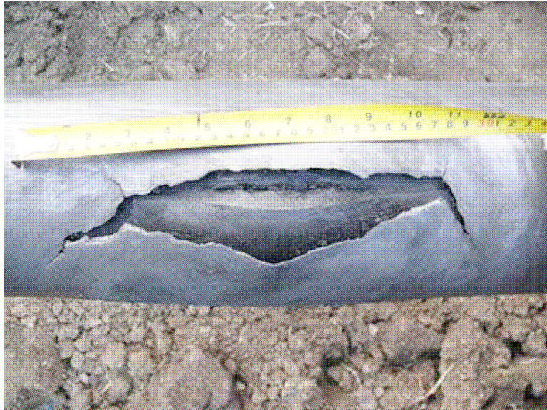
FIGURE 1 - Failure after insulation and coating removal
