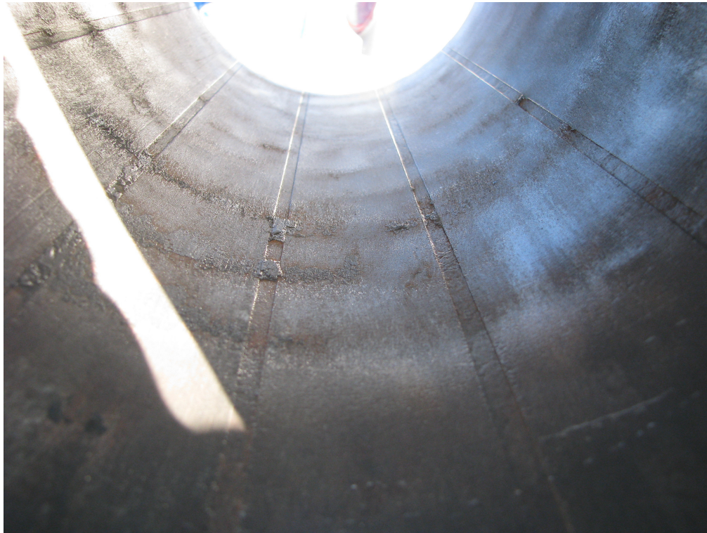
FIGURE 6 - Shallow Corrosion on Steel Pipe ID Adjacent to External Grooves in HDPE Liner
