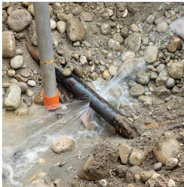
Figure SEQ Figure \* ARABIC 8. Jasper Leak
