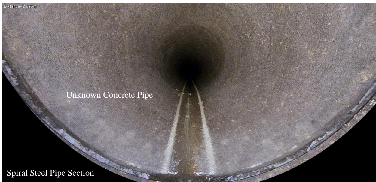
Figure 11 – Confirmation of the joint gap spacing within the video begins at 2.62m
