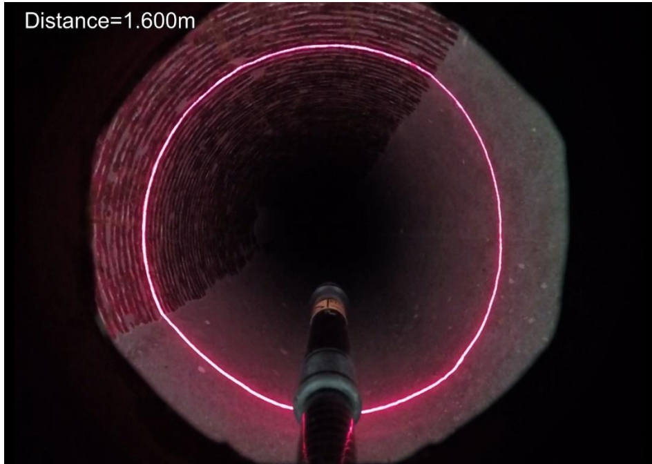
Top Image: The inspection start location at 1.6 meters shows light concrete film over the hard-facing liner on Slick Line #2
