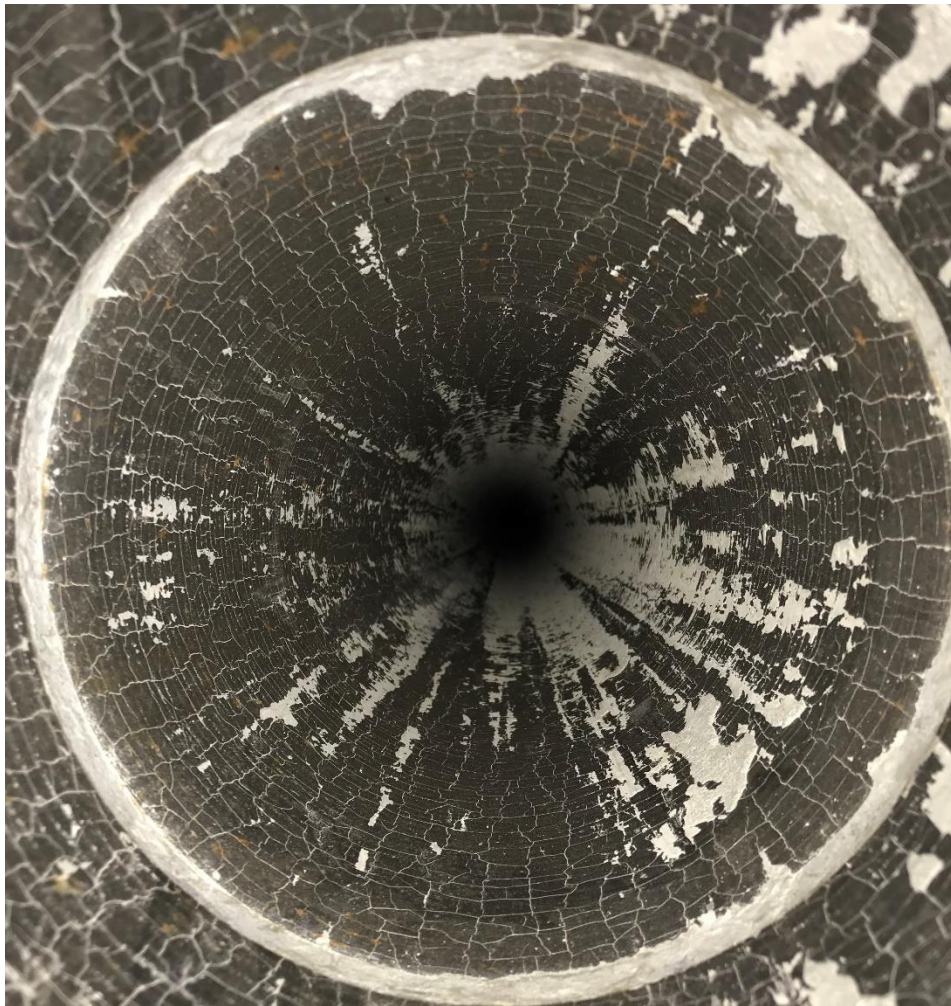
Figure 3. Both Slick Lines #1 and #2 internal hard-facing liner shows that the original weld caps have been worn smooth leaving a crazing effect. The crazing effects of the carbide liner are common to see as minor stress relief cracking during the post weld cooling process.
