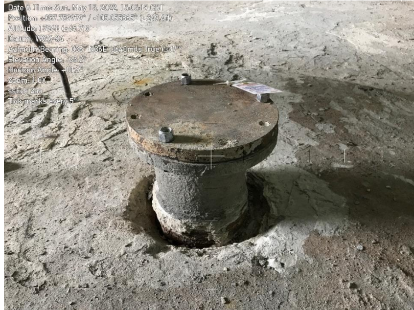
Figure 6. Slick Line 1 access with bolted flange
