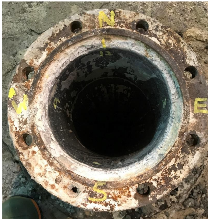
Figure 7. The Slick Line flanges and pipe walls were marked up to help reference the clock positions for when the laser inspection tool was inserted
