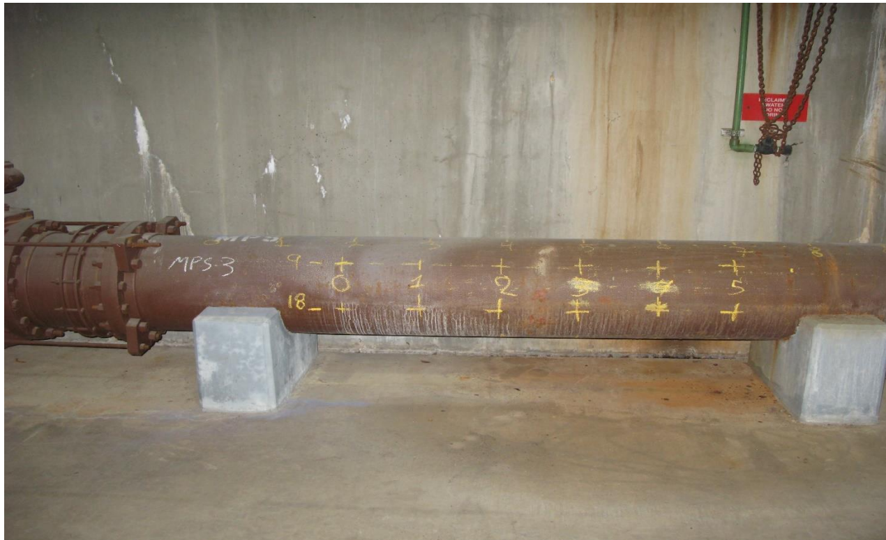
The pictures above show an example of the 18" MPS – Mixing Pump Suction piping.
