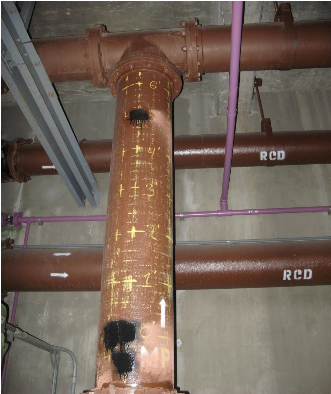
Figure A1. The picture above shows an overview of the pipe.
