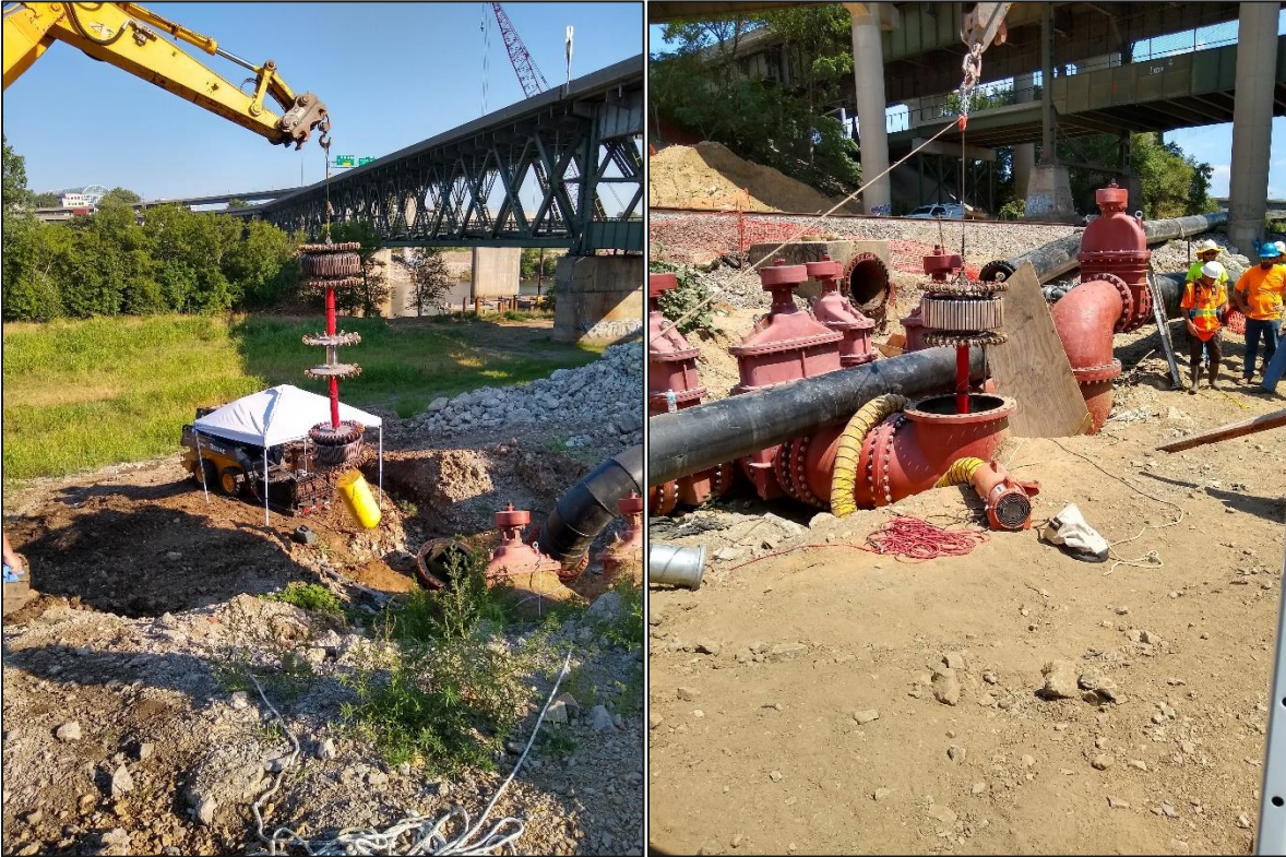
Figure 4a (left): PICA’s Chimera is lowered into the launch wye of the South line; 4b (right): the Chimera is removed through the vertical tee of the South line at the end of the inspection.
