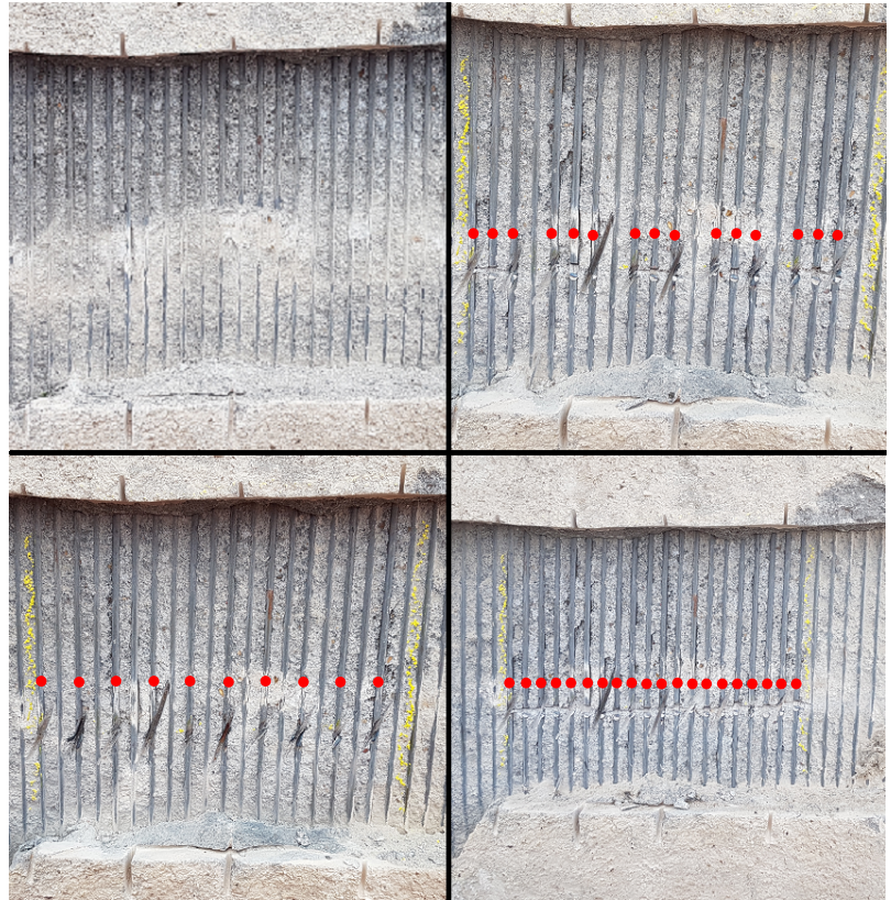
Figure 5. Exposed pre-tensioning wires
