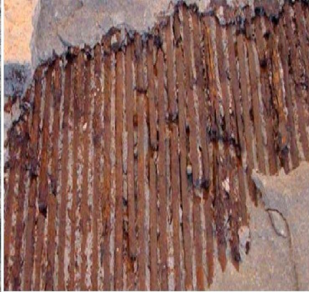
Corroded wires lose bond and recoil
